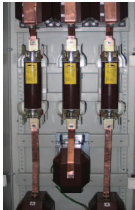
Connection in indoor switchgear, example:
